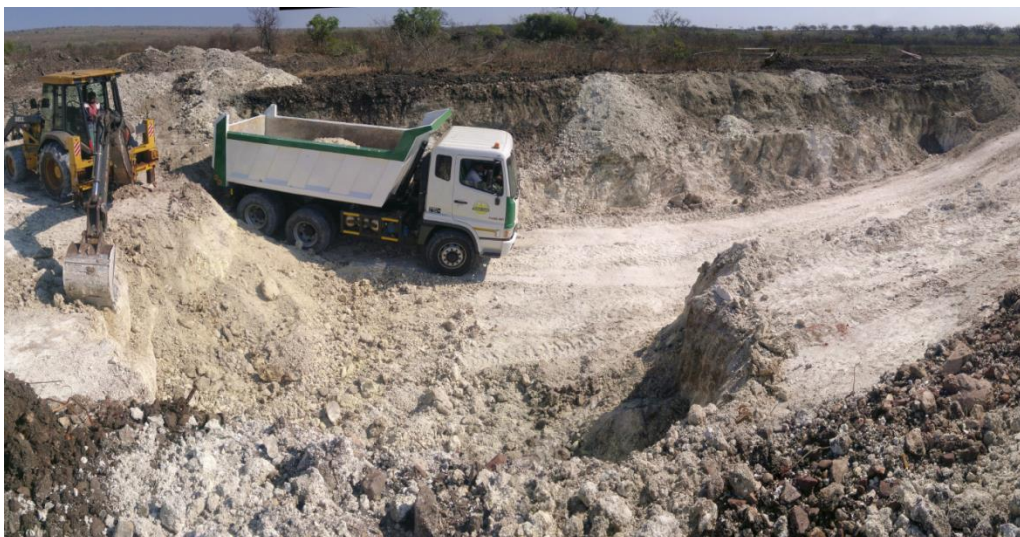
Figure 11 Trial mining of calcium bentonite at Namaacha Mining's project in Mozambique Source: Namaacha Mining
